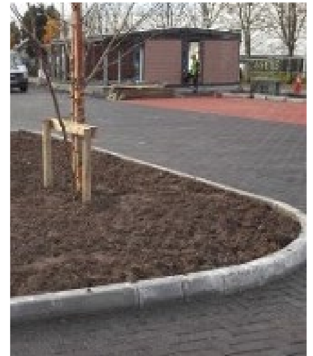
Soft landscape areas are set below kerb level at this permeable paving installation. Almac Car Park, Limerick, Ireland.
