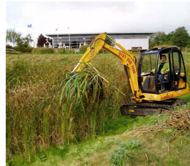
A light tracked excavator removes aquatic vegetation to de-water next to the wetland, before moving to a wildlife pile.
