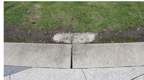
Image shows topsoil washout. The haunching is set near the top of kerb allowing for minimal topsoil to be placed, therefore prone to erosion over time.
