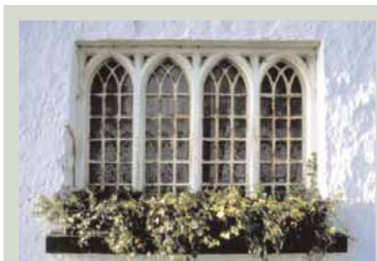
Most cast iron or steel windows contain timber sub-frames, or transoms as in this window. Sometimes the framing materials are not obvious until paint comes away and the material starts to deteriorate. It is vital to identify the framing materials when repairs are being planned
