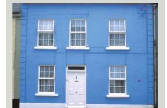
Possibly with the best of intentions, they were taken out and top-hung uPVC casements fitted instead. When closed these appear flat and insubstantial, and when swung open the superficial likeness to traditional windows is lost
