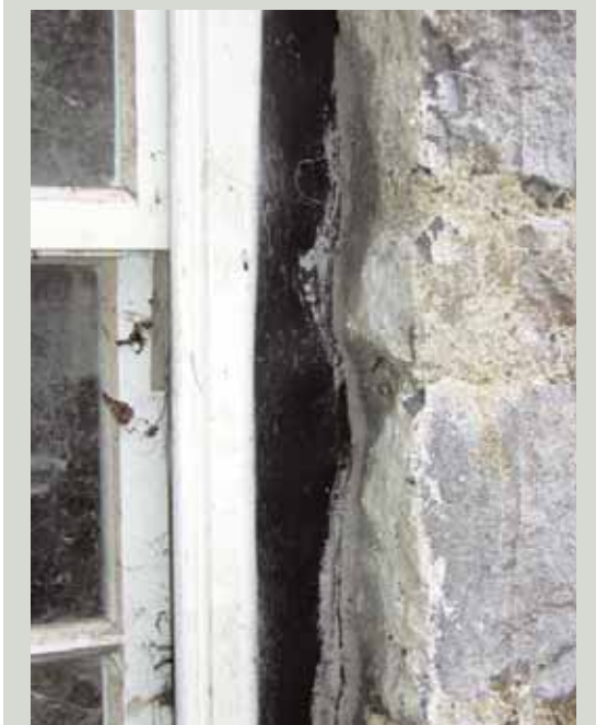
The silicone-based mastic used here is starting to lift in places, just a few years after being applied. As it is black and applied thickly it is more visible than caulking or pointing should be
