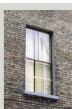
The lower sash has been removed for repainting and the opening is protected by fitting a lath across the frame and closing the shutters. It is important to prevent access to dangerous openings during a painting job
