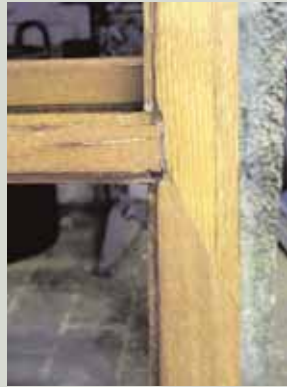
This oak sash has been repaired with new timber scarfed in, which matches the grain density and direction of the original. The repair is of high quality and should last indefinitely
