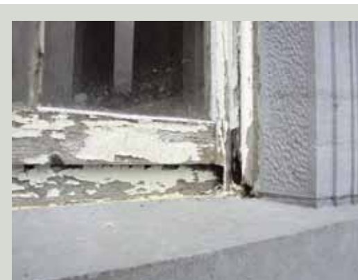
The loss of paint should not be the main guide as to the condition of the timber. Despite years of neglect, this window did not require substantial replacement of timbers. The ends of the box frame and its linings, as the most vulnerable areas, did require new scarfed repairs
