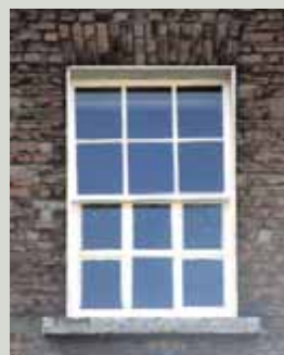
Over-cautious sealing of the putty by painting very far onto the glass can affect the appearance of the window, especially if it is not done consistently
