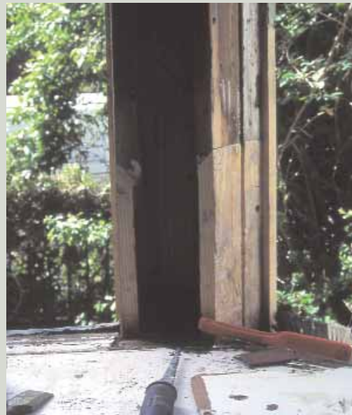
Previous repairs to the ends of this mullion were uncovered during a refurbishment project. The repairs remained in good condition and did not need attention
