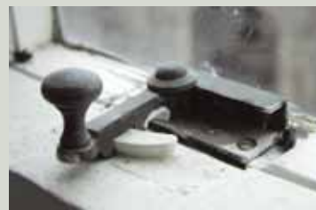
The meeting rails must line up accurately for quadrant fasteners to close properly, as was done when this window was repaired
