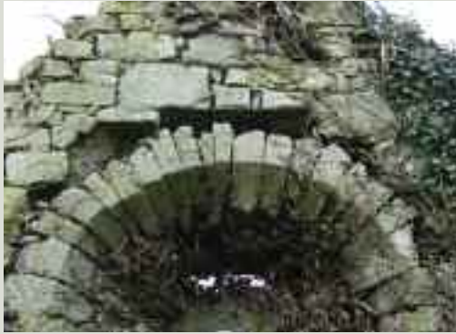
Arch over a window. Note the damage done by the improper removal of ivy which pulled out the smaller packing stones and has left the arch vulnerable
