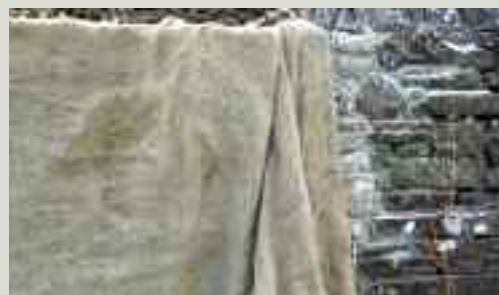
Protective hessian on masonry work is far more effective than plastic sheeting and can be reused many times
