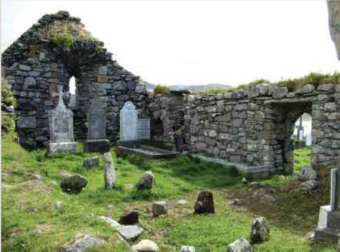
Graves close to a ruined church wall can damage the masonry foundation itself and undermine the earth supporting the foundation
