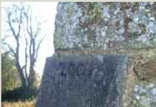
A date has been etched into the stone to distinguish the new stone from the original
