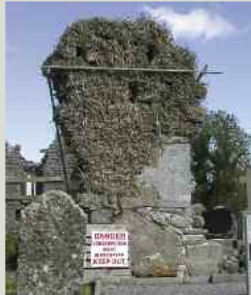
A clear sign warns of conservation works in progress. The temporary works to the wall in the background include scaffolding poles to provide restraint. The concrete blockwork on the right hand side provides temporary propping pending reinstatement of the wall core
