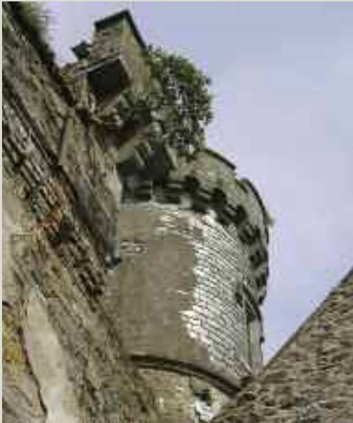
While more commonly found as a roofing material, slate was also used as a cladding material for exposed walls, gables and chimney stacks. The slates found in slate-hanging are often rare examples of native Irish slates which, because of their small sizes, were often replaced on roofs by Welsh slates
