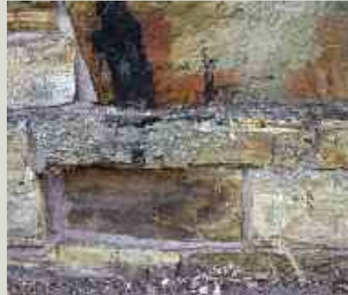
Delaminating stone, bedded vertically
