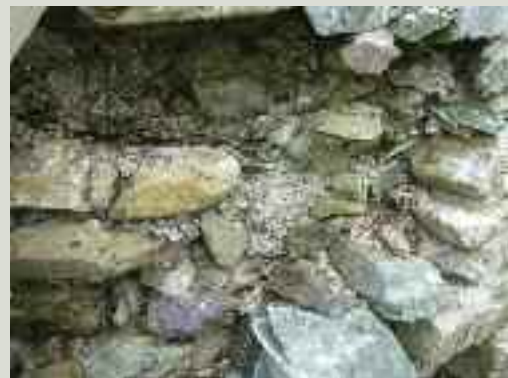
Wall with its outer face lost exposing the construction of the wall core
