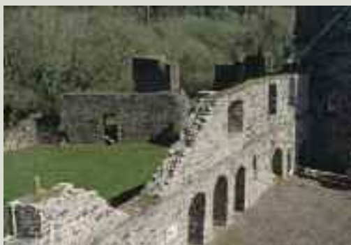
Flaunching, a sloping area of mortar, has been applied to the raking surface and also to the upper surface of this wall on which a mat of vegetation is beginning to grow
