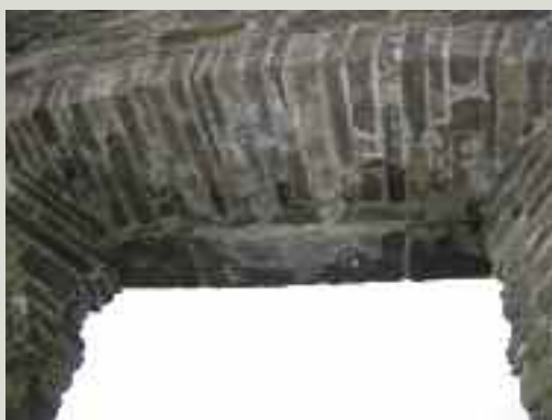
Failed lintel with stainless steel rods used to carry out a stitch repair
