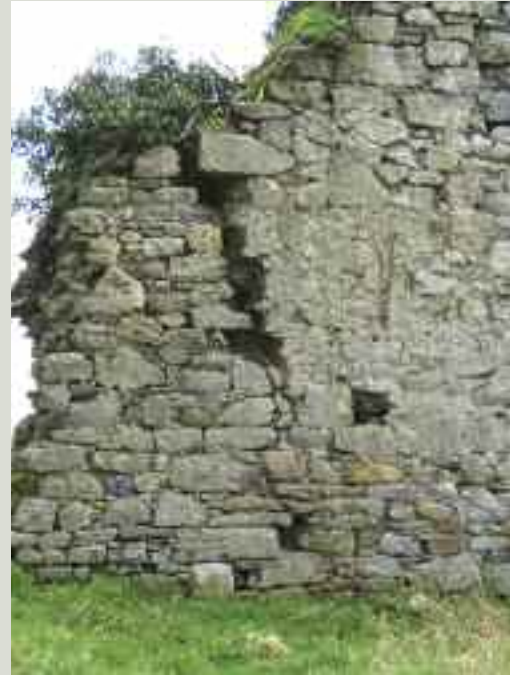
Tapering cracks can result from subsidence. As the crack widens the smaller stones fall out or drop inside the wall creating a wedge effect and increasing the damage
