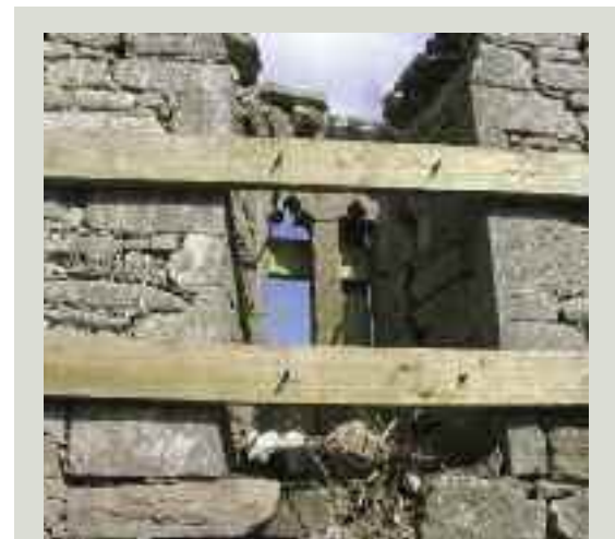
Timber bracing in the vertical plane to secure a window opening where a collapse outwards was imminent. The temporary work consisted of planks bolted through the opening
