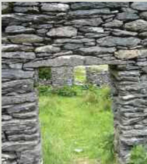
Stone lintel over a narrow opening. The thinness of the lintel, particularly at the right-hand end, makes it vulnerable to cracking
