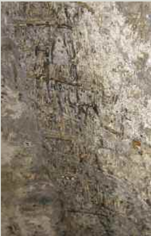
In this example of wicker centring on the underside of a vault, not only the imprint of the wickerwork but also parts of the original wicker matting itself have survived embedded in the mortar layer
