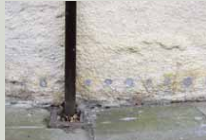
The drill holes associated with injecting a chemical DPC can be unsightly. A more effective method of dealing with the damp problem in this case would have been to reduce the level of the impermeable paving around the building and ensure that rainwater drains away from the base of the wall
