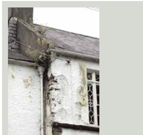
Damp problems in ground floor or basement rooms may not be caused by rising damp but by rainwater from broken gutters above saturating the wall and the ground beneath
