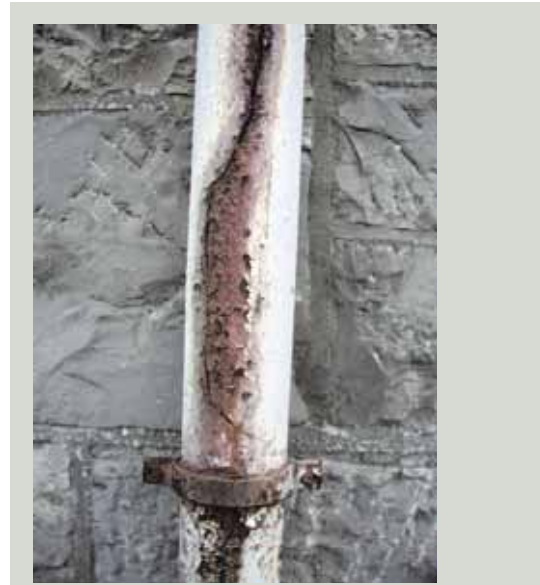
Iron rainwater goods such as gutters, hopper heads and downpipes are extremely long-lasting if given regular and frequent painting to prevent corrosion. Where they have already started to rust, the iron should be properly prepared before repainting
