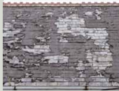
Covering a leaking roof with a coating of bitumen or mineral felt may seem to provide an easy solution but, as well as its unsightly appearance, it is not long-lasting, will make it difficult to trace the source of any future leaks and will hinder the reuse of the original slates for reslating the roof
