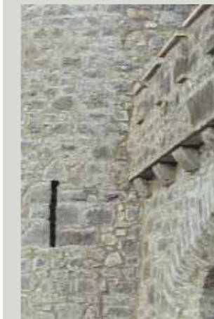
Dealing with structural cracking in walls requires specialist advice. Cracks can be successfully repaired once the cause of the structural movement has been identified and the problem solved
