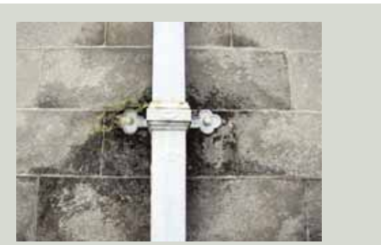
The staining of the stone wall behind this downpipe joint suggests there is a blockage inside the pipe. If the water trapped inside freezes in cold weather, it may burst the pipe
