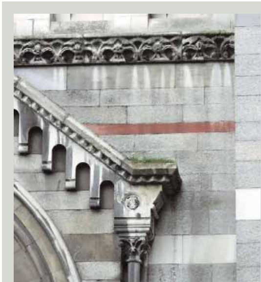
Parts of a building may be difficult to access and are likely to be neglected for that reason. Plants have begun to take root on this high level decorative detail and should be removed before they cause damage to the fine stonework
