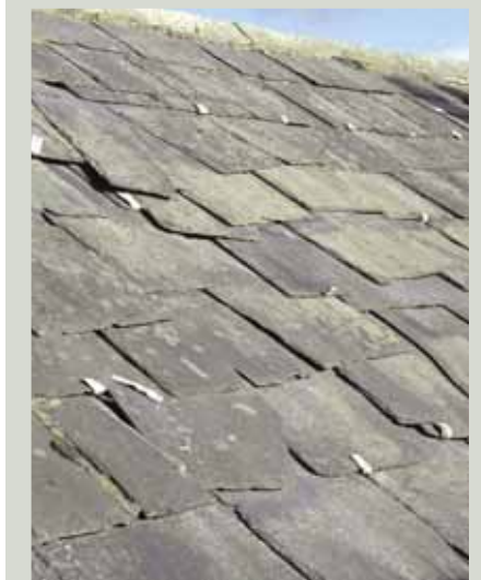
A number of tingles have been used in previous repairs of this roof but the slipping of slates continues, indicating a widespread failure of fixings. As a rule of thumb, where a third or more of slates have slipped the entire roof will require to be stripped and re-fixed, reusing the existing slates where possible
