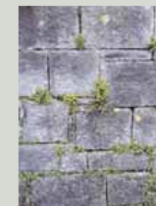
Although the plants which have taken root between the stones of this boundary wall may be visually attractive, they are a clear sign that the mortar has decayed over a widespread area, water is lodging within the wall and action is needed
