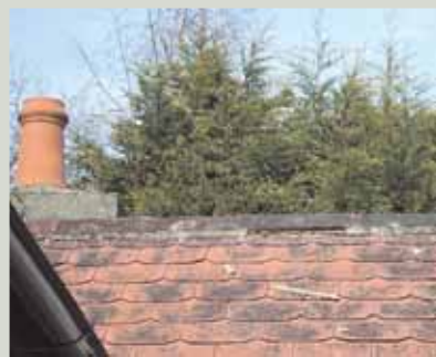
The mortar used to fix ridge tiles in place should be inspected to ensure that it has not become loose or detached
