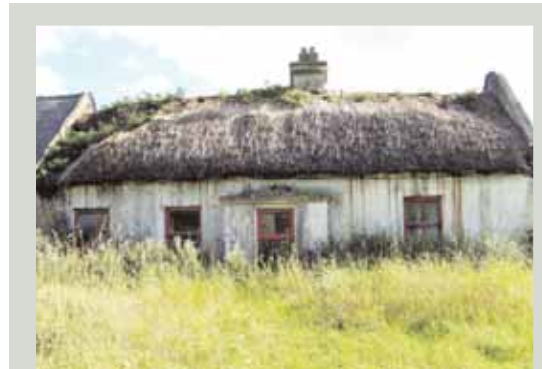
The condition of thatched roofs can deteriorate rapidly if not kept in good repair
