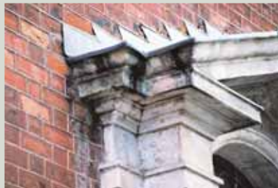
It may sometimes be necessary to add flashings where none originally existed if it is clear that damage is being done
