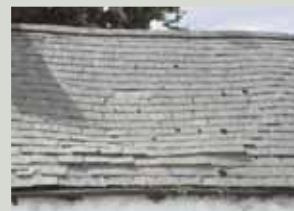
This roof is showing signs of sagging which probably indicates decay or damage of the structure beneath which must not be ignored
