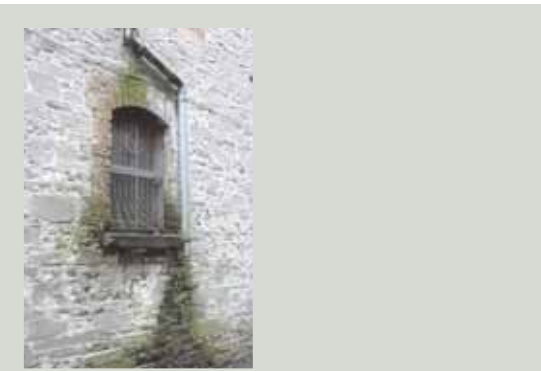
Leaking joints and missing sections of downpipe are relatively cheap and easy to fix if attended to promptly. When defects are not remedied, they lead to serious problems which are expensive to repair and involve the loss and disruption of parts of the building fabric
