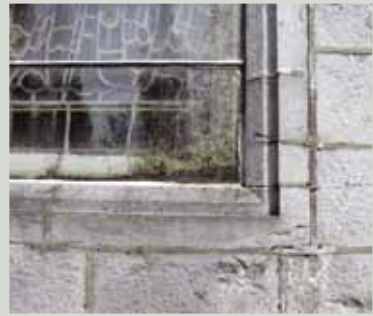
Poor ventilation of the space between a stained glass window and new storm glazing has created so much condensation that plants can now grow which will damage the stained glass panel
