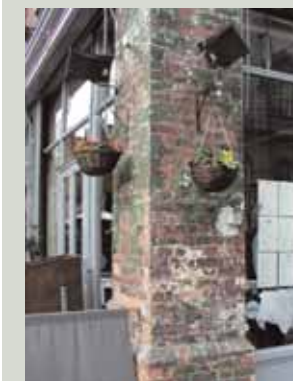
Painting brickwork or stonework as a short-term solution to cover over defects is not advisable. Applying impermeable paints will make most problems worse and the coatings are difficult, or impossible, to satisfactorily remove later without damaging the wall beneath
