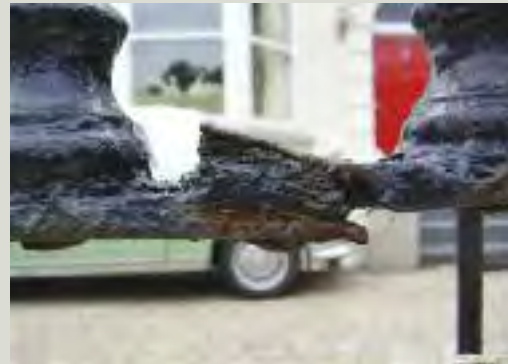
Corrosion developing at a scarf joint
