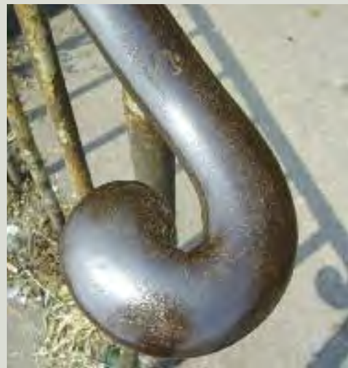
An oxide layer has developed on this wrought iron handrail which protects it from further corrosion
