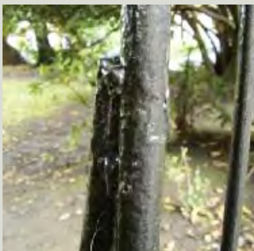
This backstay has been repaired by welding it back into position, which is not in keeping with the traditional techniques used to assemble this railing
