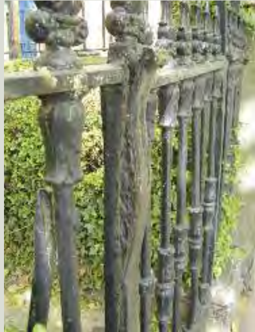
Corrosion between the gate frame and slam bar is common
