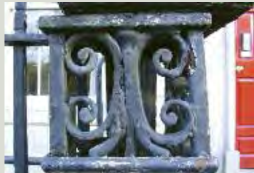
Posts from two different properties on Parnell Square, Dublin. While appearing to be severely corroded, much of the original ironwork in the lower example may remain intact beneath layers of paint and corrosion
