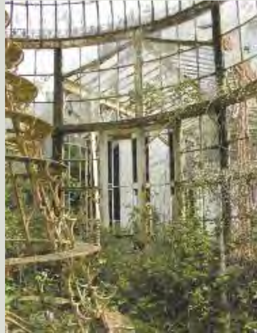
This finely-made circular conservatory was designed and erected at Castlebridge House, County Wexford by James Pierce of Mill Road Iron Works, Wexford. In addition to its iron structure, it contains a 10-tier iron display stand for plants at its centre
