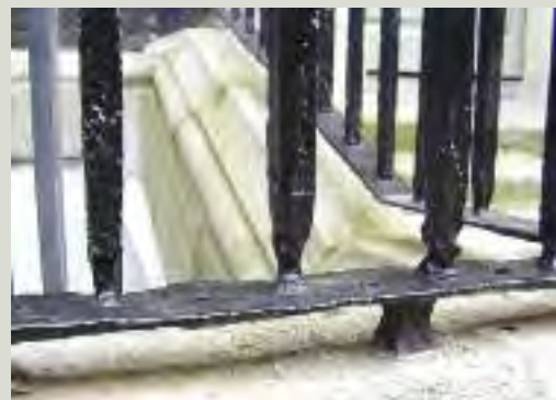
Bars do not necessarily need to be replaced when they have wasted at their base. Unless their condition is compromising the integrity of the ironwork, they can be left in place
