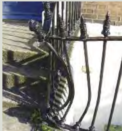
Impact damage caused for example by vandalism or cars, can cause deformation (in the case of wrought iron) and fracturing or shattering (in the case of cast iron)
