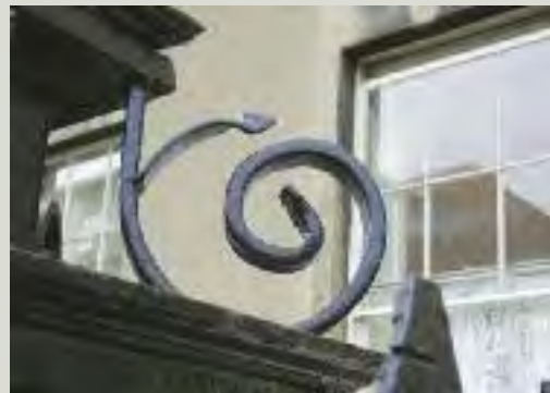
It is important to choose an experienced craftsman to avoid inappropriate repairs. The replacement scroll in the lower image has been crudely formed and bears little resemblance to the finely-crafted original feature on a neighbouring property in the top image
