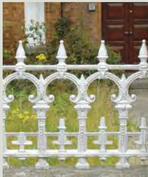
This design is typical of cast iron panels cast in repeating, identical sections. Patterns for railings such as these had to be designed so that there were no undercuts – it had to be possible to pull the pattern out of the sand mould without pulling away any of the sand (which would get trapped behind undercuts) in the process. Some panels have a taper from one side to the other which aided the removal of the pattern from the sand mould
