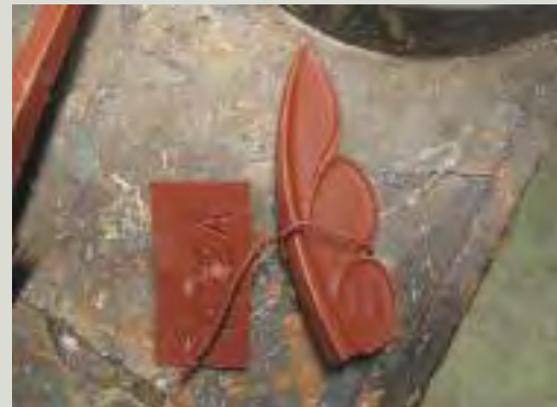
Attaching metal tags to ironwork as it is dismantled (numbered to correspond with a measured survey drawing) is essential for tracking repairs and for correct reinstatement (Image courtesy of Historic Scotland)
