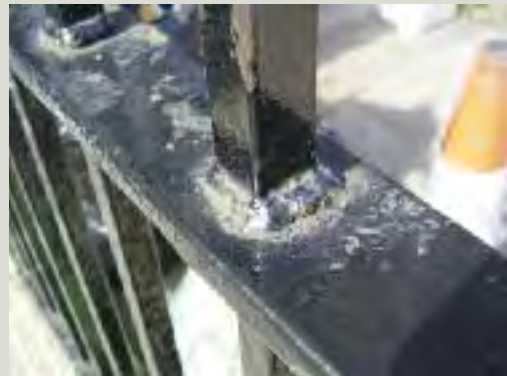
Poorly-finished weld joints can be disfiguring to traditional and new iron and steelwork alike
