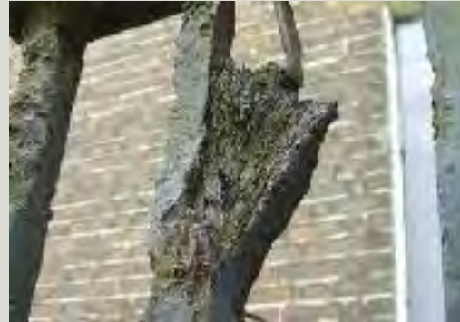
Wrought iron typically 'delaminates' as it corrodes, accentuating the fibrous structure of the material
