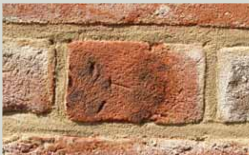
Remedial work in the form of a quality pigmented mortar repair. It shows that, when necessary, and executed with great skill, a mortar repair can provide a temporary repair that achieves the desired effect
