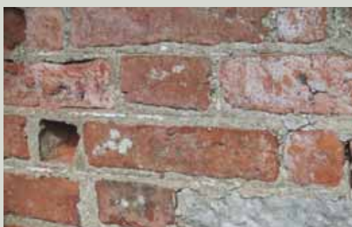
Colour washed bricks with traces of pencilling to the joints at the Hell Fire Club, Desmond's Castle, Askeaton, Co. Limerick
