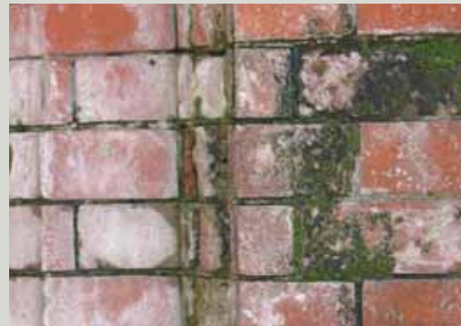
Soluble salts visible on the surface of this brickwork have been caused by rising damp in the wall. The moss growth present is another symptom of the excessive dampness of the bricks the cause of which needs to be diagnosed and treated
