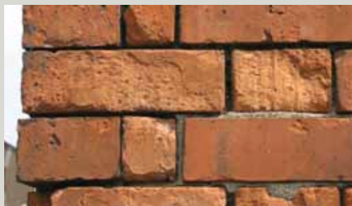
The mortar has weathered back or been washed out of this brickwork to a severe extent and it is now in urgent need of repair and repointing
