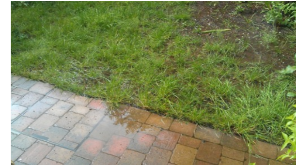
Image: water logged courtyard
