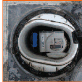
Blue Isolating Valve within Meter Box
