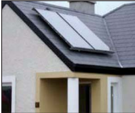
Example of solar panels on an extension.
